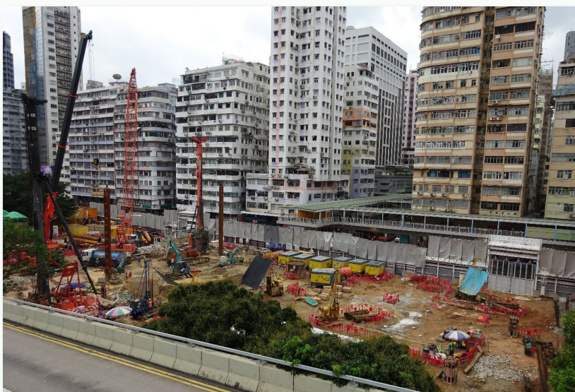
▲ New measures are in place on a site at the junction of Sai Yee Street and Argyle Street, Mong Kok to foster a quality and sustainable built environment there.
